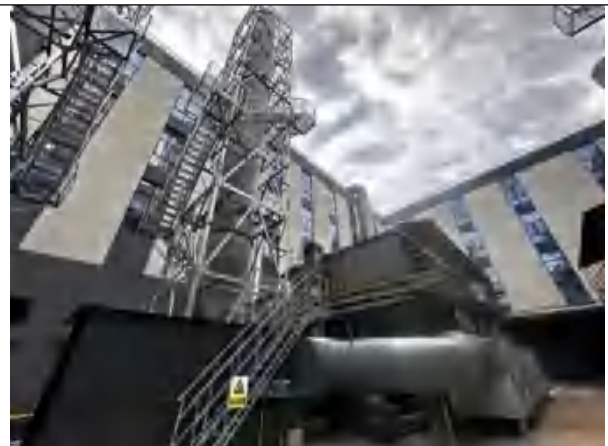
DA011A 线 RTO 排气筒及走梯
