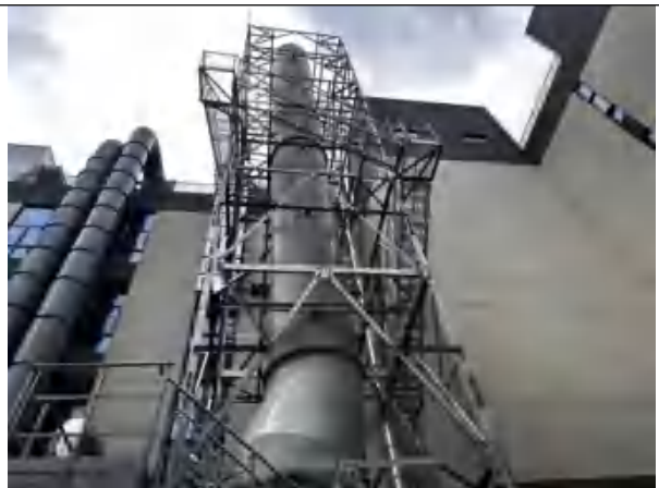
DA012 沸石转轮废气排气筒及走梯
